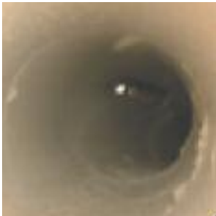
Internal section of a transfer pipe showing perforations of both the internal lining system and the outer steel casing
