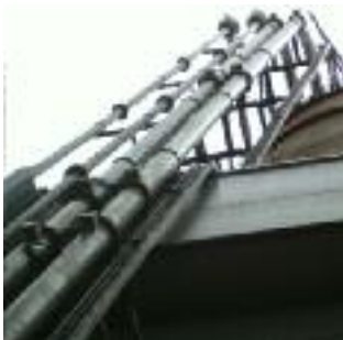
Arrangement of a cluster of pipes incorporating the AbrAlarm system fitted in position and being hardwired back to a remote control system
