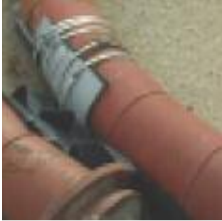
Example of a pipe that has perforations on the steel casing showing an attachment of a temporary patch preventing material escaping to atmosphere
