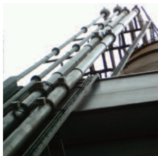
Arrangement of a cluster of pipes incorporating the AbrAlarm system fitted in position and being hardwired back to a remote control system
